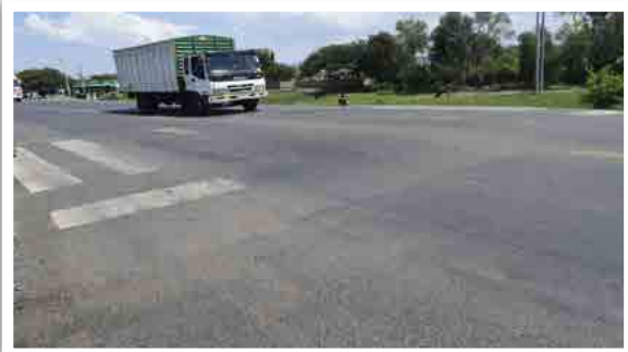
Figure 27: Faded road markings at a pedestrian crossing
