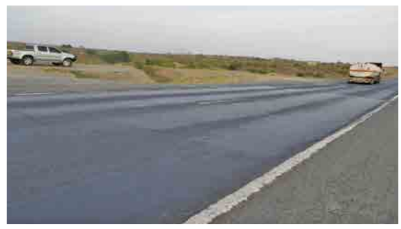
Figure 11: Bleeding road surface
