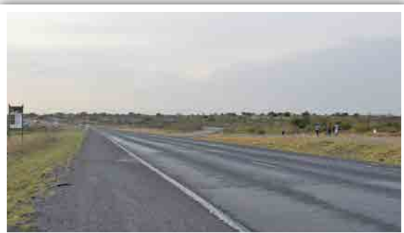
Figure 12: Deep open drains too close to the carriageway
