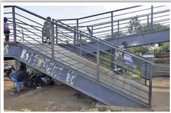
Figure 34: An abnormally steep ramp on the footbridge
