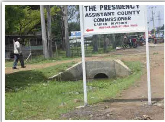
Figure 31: Silted/blocked access culvert
