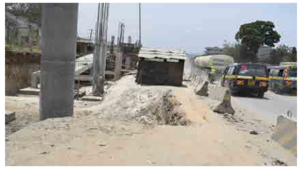
Figure 5: Site management concerns at the ongoing footbridge construction (Unsecured excavation)
