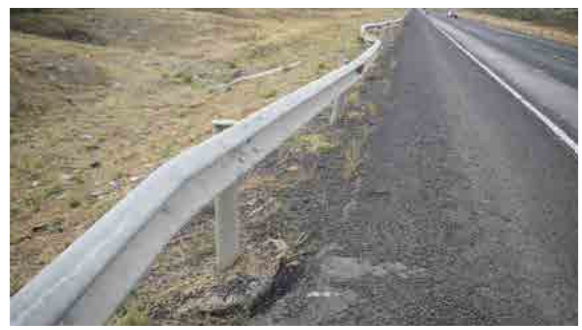
Figure 13: Damaged safety fences/guard rails
