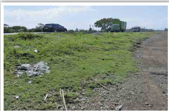
Figure 29: Missing safety fences on a high steep-sloped embankment
