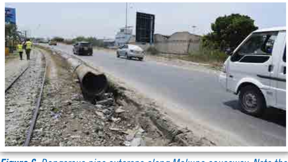
Figure 6: Dangerous pipe outcrops along Makupa causeway. Note the close proximity between the carriageway and railway line
