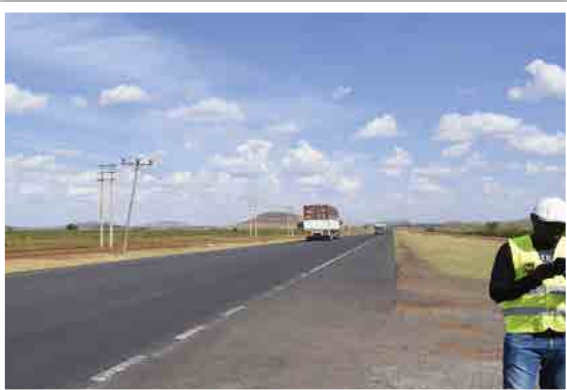
Figure 16: Long and straight stretch along Pipeline area. Faded road markings at the stretch also observed
