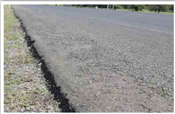
Figure 28: Hanging road shoulders
