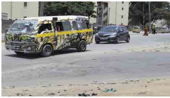
Figure 3: Deteriorated road surface at Makande Junction
